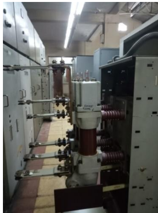
Gambar 5.4 Oil Circuit Breaker
