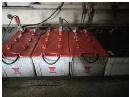
Gambar 4. 1 Battery Starting Generator
