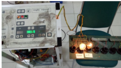
Figure 7. Condition of the Exposure Tool
