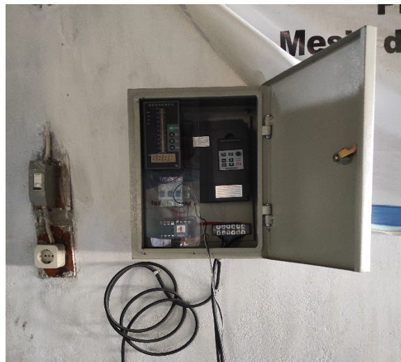
Gambar 7. Power inverter DC-AC terpasang.
