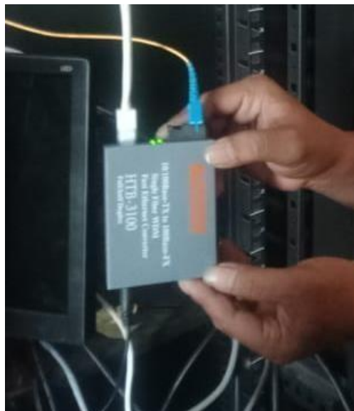
Gambar 4.8 HTB Kabel FO Pengirim
